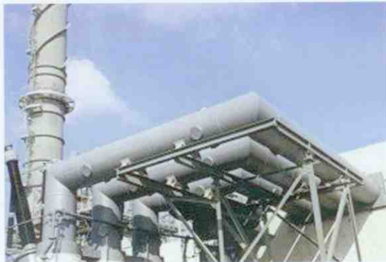
伊朗阿拉克电厂 Arak Thermal Power Plant in Iran
